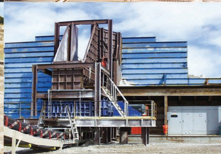
Gypsum | USA | In: ROM | Out: -250mm | Capacity: 1,000TPH
