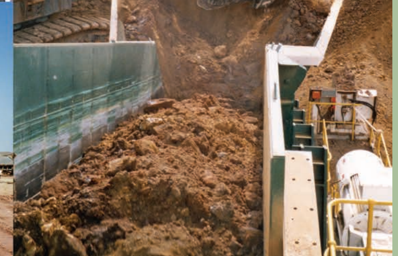
D9 Apron Plate Feeder with electro-mechanical drive
